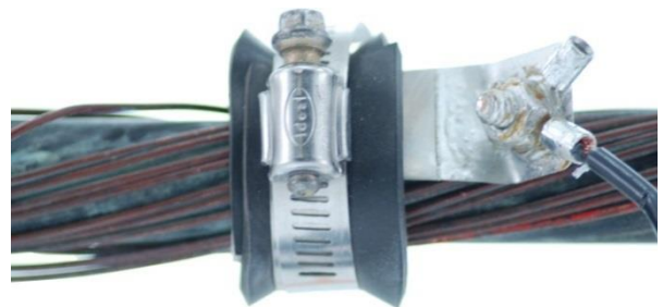
Figure 5: Neutral clamp attached to the new copper.
