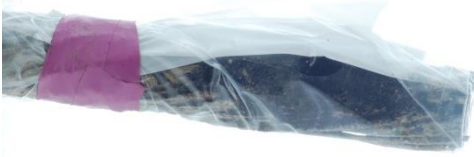
Figure 8: Sealed cable ends.
