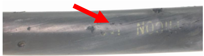
Figure 5: Pits caused by rodents chewing on the cable.
