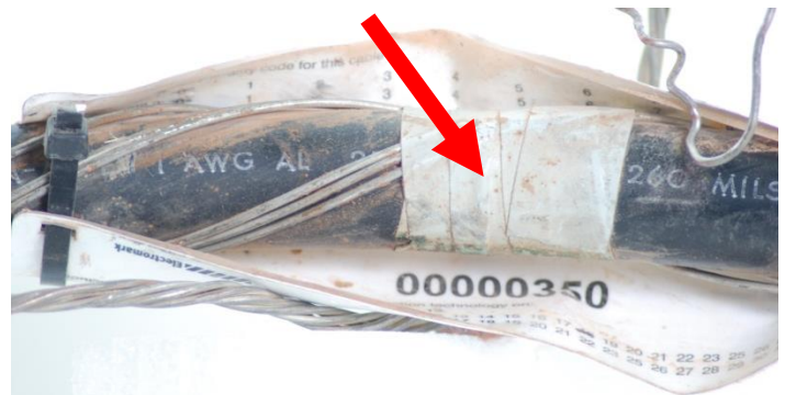
Figure 3: Bare neutrals secured with vinyl tape.
