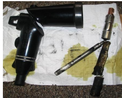
Figure 7: Damaged components have been removed.
