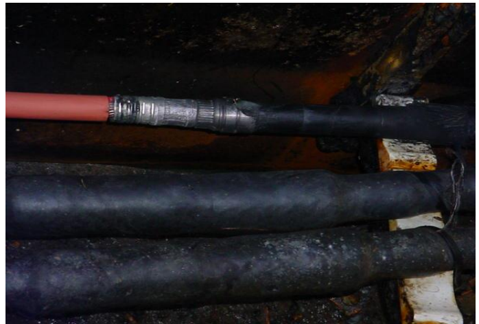
Figure 10: The re-jacketing sleeve and splice were removed without marking tape, making it impossible to know for sure if the splice had been centered. With a lot of hard work it was still possible to determine that it was not centered properly.
