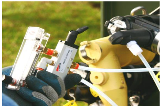
Figure 10: Perform flow test to verify that adequate flow exists through the cable system before injection.
