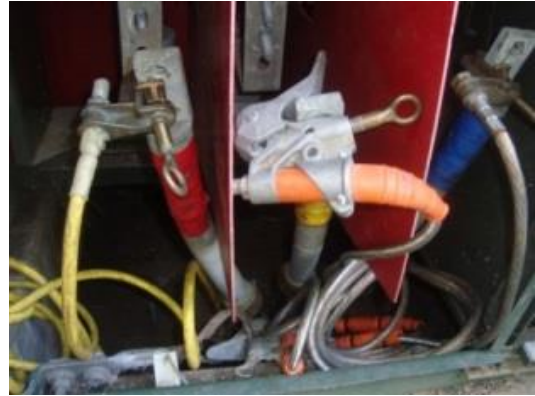
Figure 3: Use the HIDD to ground the cable softly to bleed off the capacitive charge before installing the safety ground.
