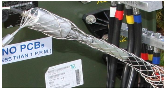
Figure 3: Use an ITD to streamline the TDR signal as it transitions into the cable.
