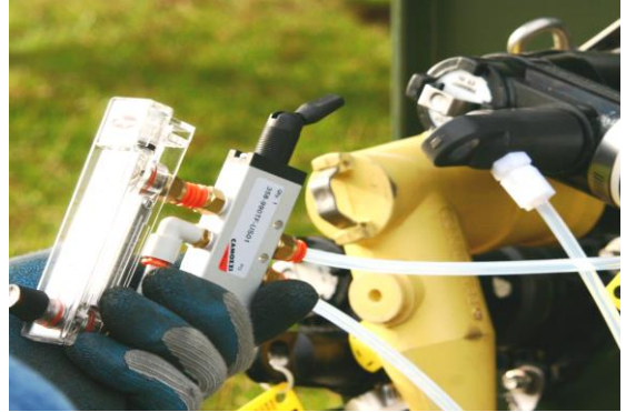
Figure 8: Perform flow test to verify adequate flow exists through the cable system prior to injection.
