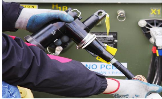
Figure 6: Install injection terminations and perform termination test to identify leaks and blockages.
