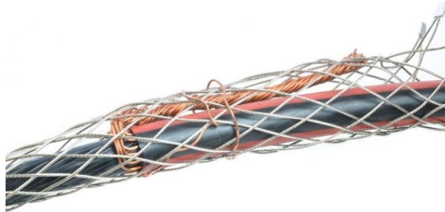
Figure 4: The ITD Streamliner's Kellems grip in good contact with the neutral wires.
