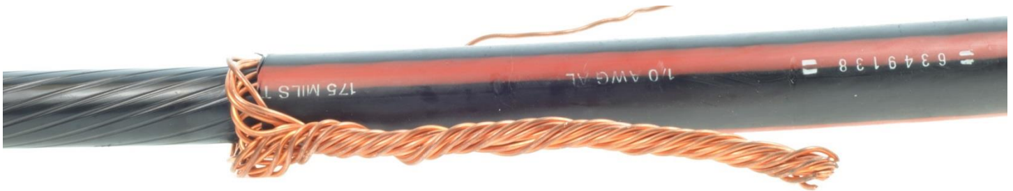
Figure 1: Winding the neutrals together can help minimize separation to the conductor.
