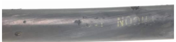
Figure 3: Damage to the semi-con.
